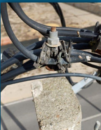
Aerial network connector damaged
