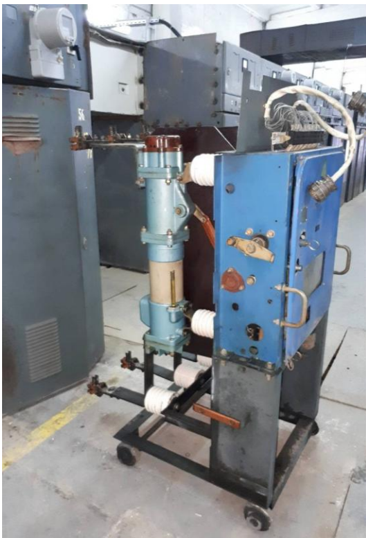
Before: Oil circuit breaker
